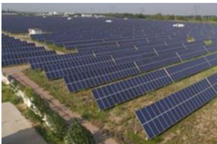
Figure 1: solar Power Plant (Dengkou, right photo).
